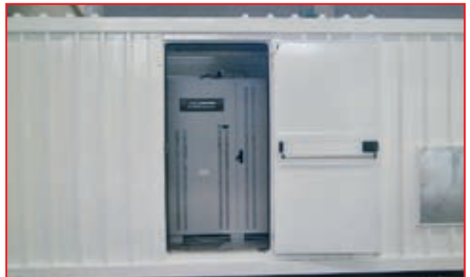
UPS mounted in a shelter
